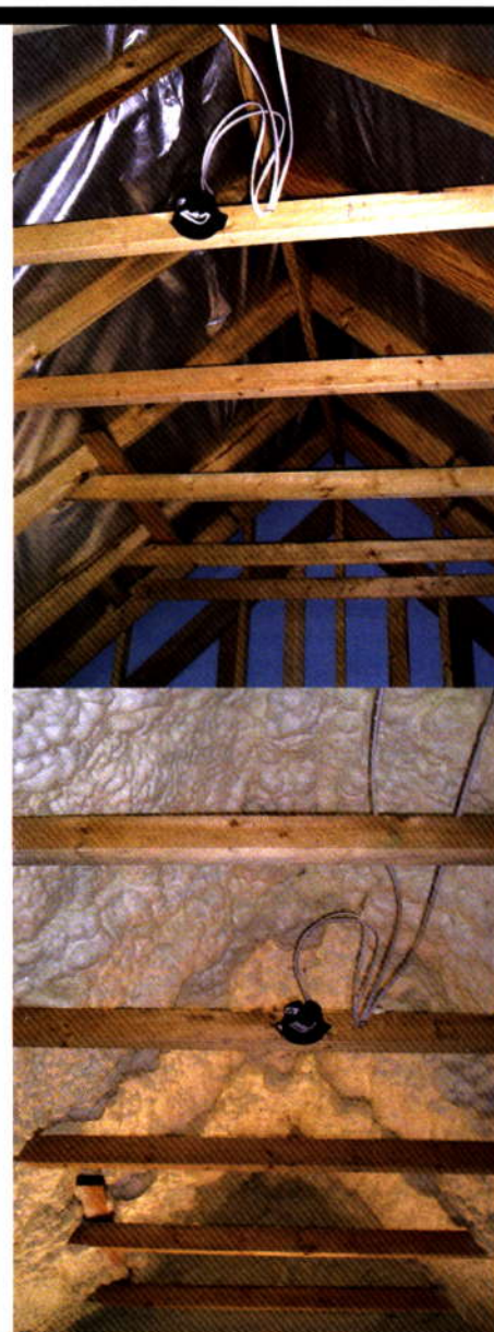
Before and after spray foam insulation was installed in this attic space for a tighter building envelope.
