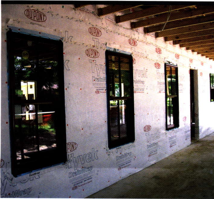
For engineering the Bannister House, Chris Miles of GreenCraft Builders used a tyvek wrap on the outside that went up past the porch ceiling combined with foam on the inside. Miles says it was the tightest building envelope he has ever completed. HVAC bills for the 2400-sq.-ft. house are averaging about $45 per month.
